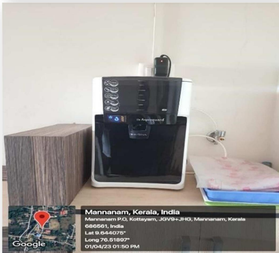
Water purifiers positioned at different parts of the college.
