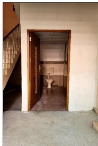
Divyangan Friendly Toilet
