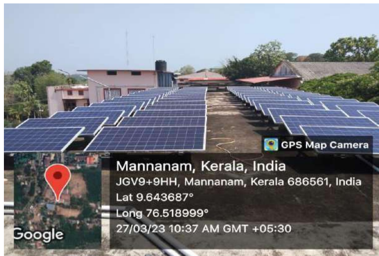
Fig. 5 Solar panel installed
