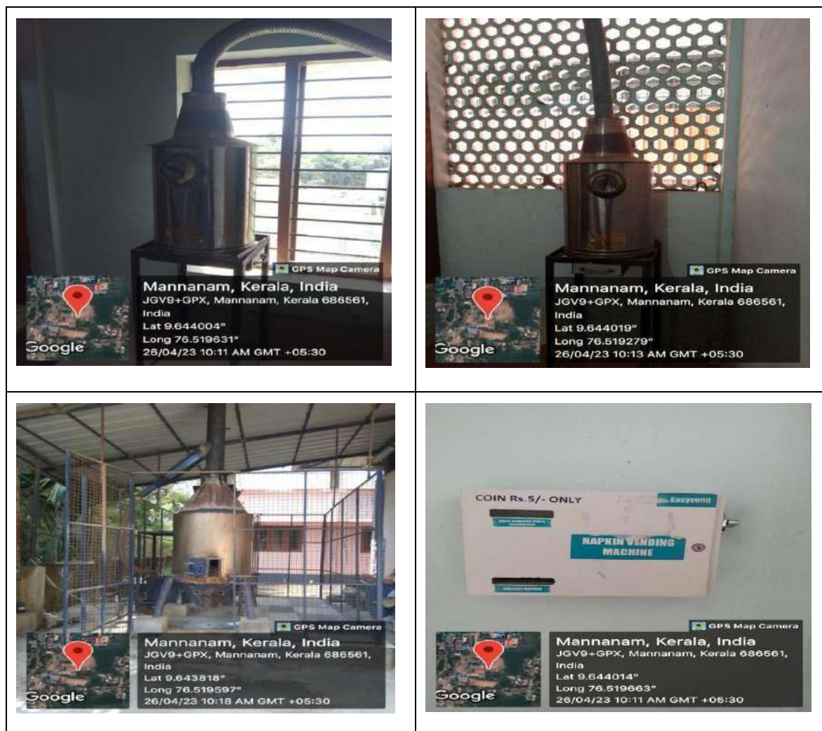
Fig. 7 Incinerators and napkin vending machine in the campus
