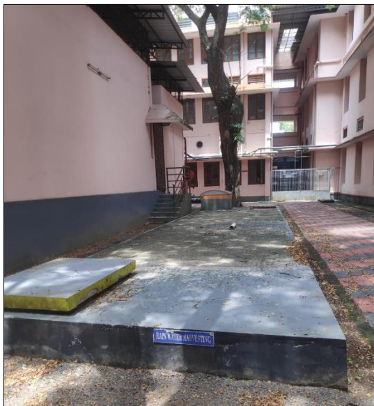
Rain Water Harvesting
