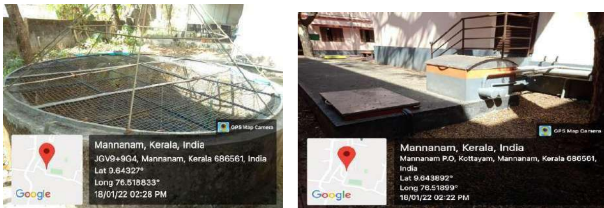
Fig. 10 Rain water harvesting structures
