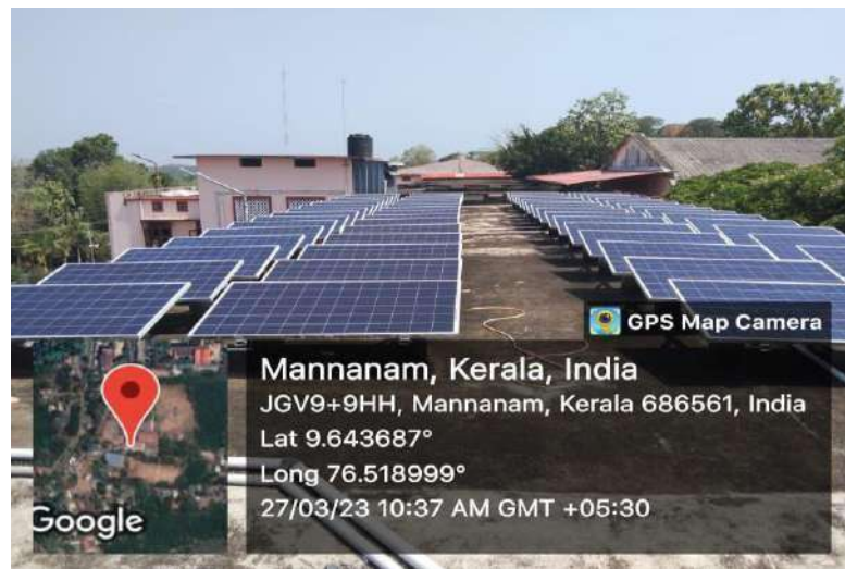
Fig. 5 Solar panel installed
