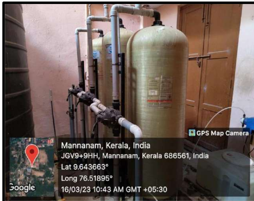
Water Treatment Plant in the Main Block
