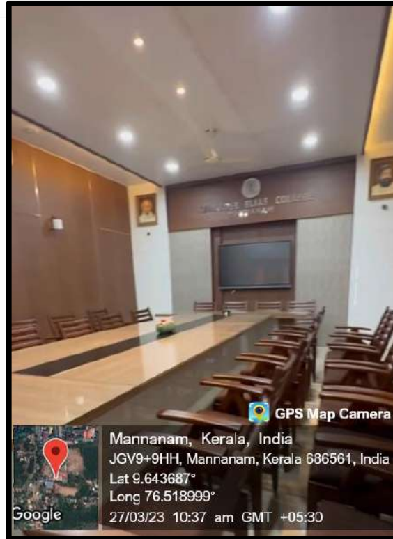
LED Lights installed at Conference Hall
