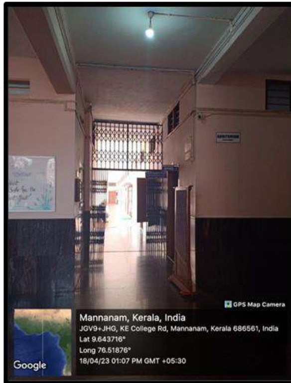
LED Bulb at Corridor of First Floor in Main Block
