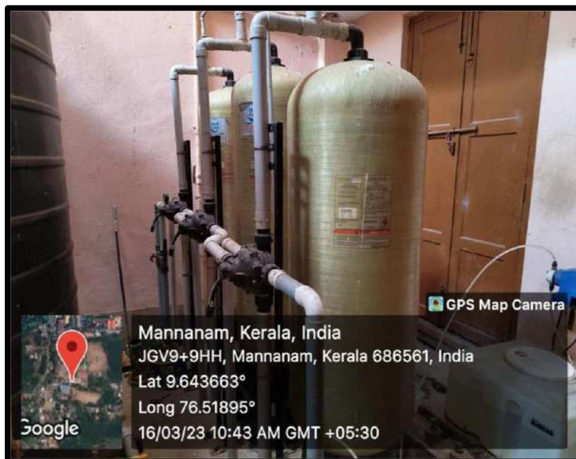
Water Treatment Plant in the Main Block
