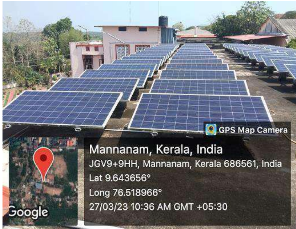
Fig. 3 Solar panel installed
