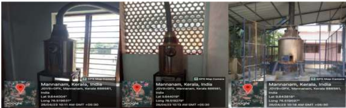
Incinerators for sanitary napkins
