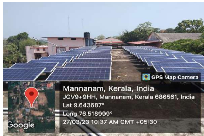
Fig. 5 Solar panel installed
