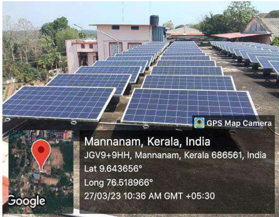
Fig. 3 Solar panel installed
